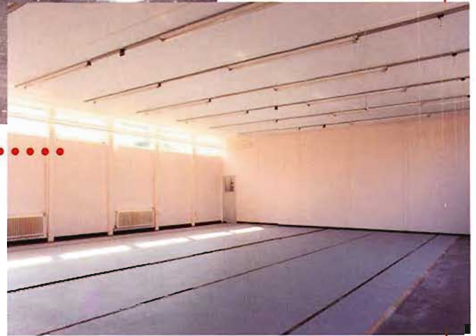
2 Rails are laid out and levelled to 1 in 1000. Once levelled, grout is applied and cured before taking load
